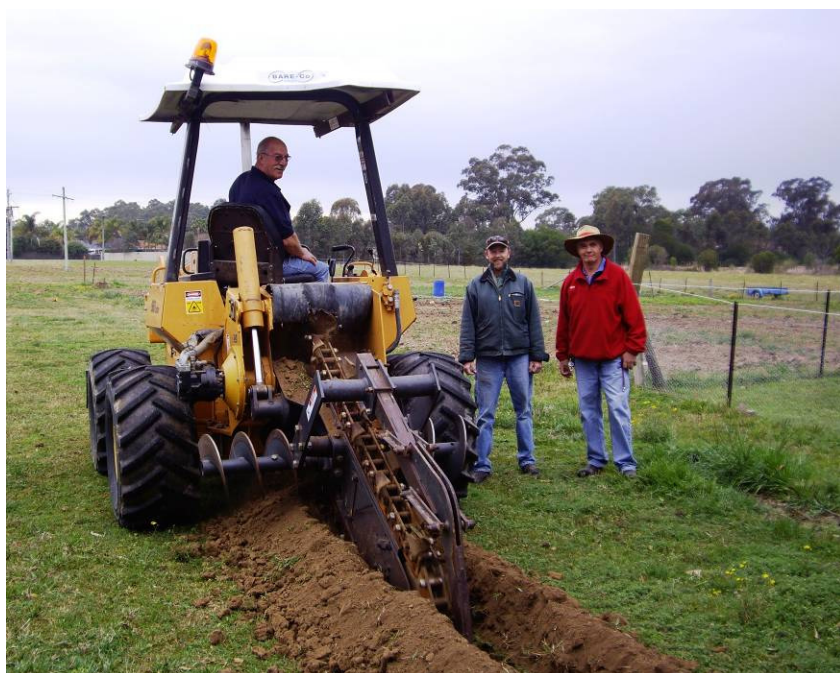
Semco's Phil Williams operates the Case trencher while Mamre Homestead's Farm Manager Luke Jewell(R) and Ian MacGregor (L) watch progress.
