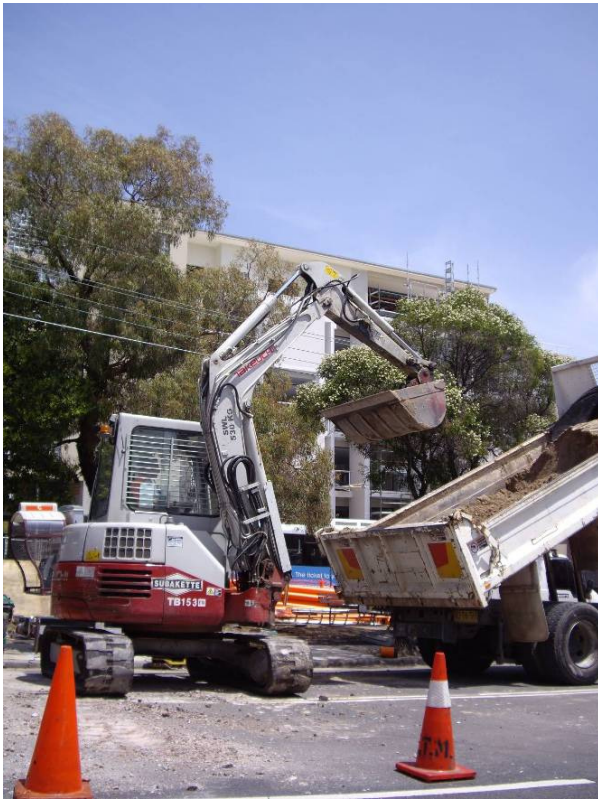
Photo: Subakette's Takeuchi zero swing excavator: full buckets for fast loading in confined spaces.
