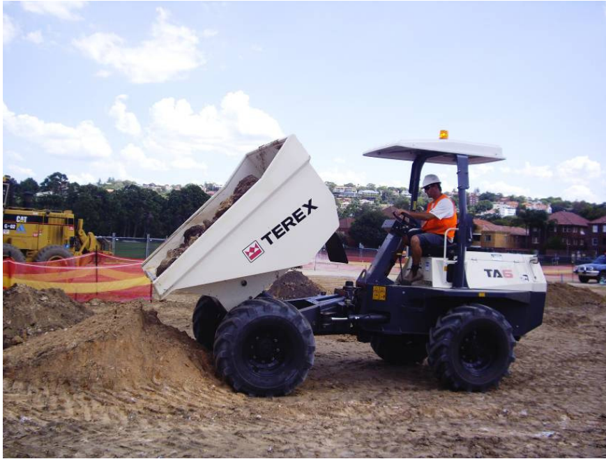
Photo: The Terex TA6 Dumper from The Watercart Specialists Pty Ltd at work on a construction site at Rose Bay, Sydney
