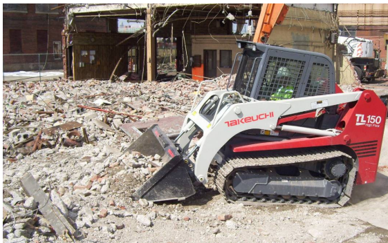
Photo: The test model Takeuchi TL150 High Flow compact loader with steel tracks undergoing testing on a demolition site.
