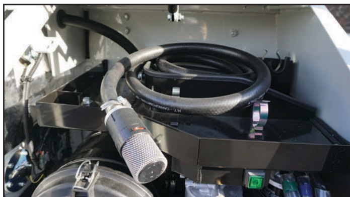
Fuel Transfer Pump
